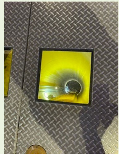
This is a picture of the 40 foot sinkhole that has been repaired, but has this very interesting view of the depth of the sinkhole.
